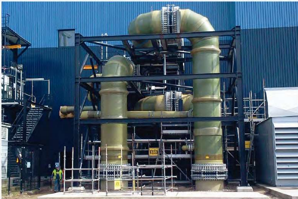
SIEMENS / HEWEG POWER PLANT, NETHERLAND 78 INCH (DN 1950) X 500mmL EXPANSION JOINT INSTALLATION VIEW
