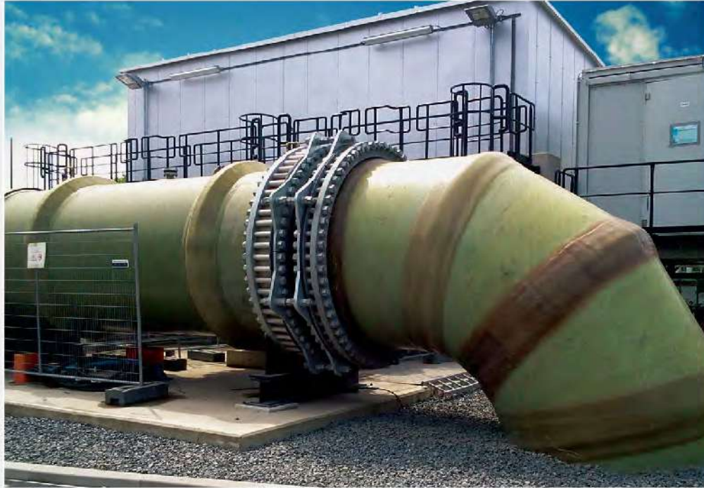
SIEMENS / HEWEG POWER PLANT, NETHERLAND 78 INCH (DN 1950) X 500mmL EXPANSION JOINT INSTALLATION VIEW
