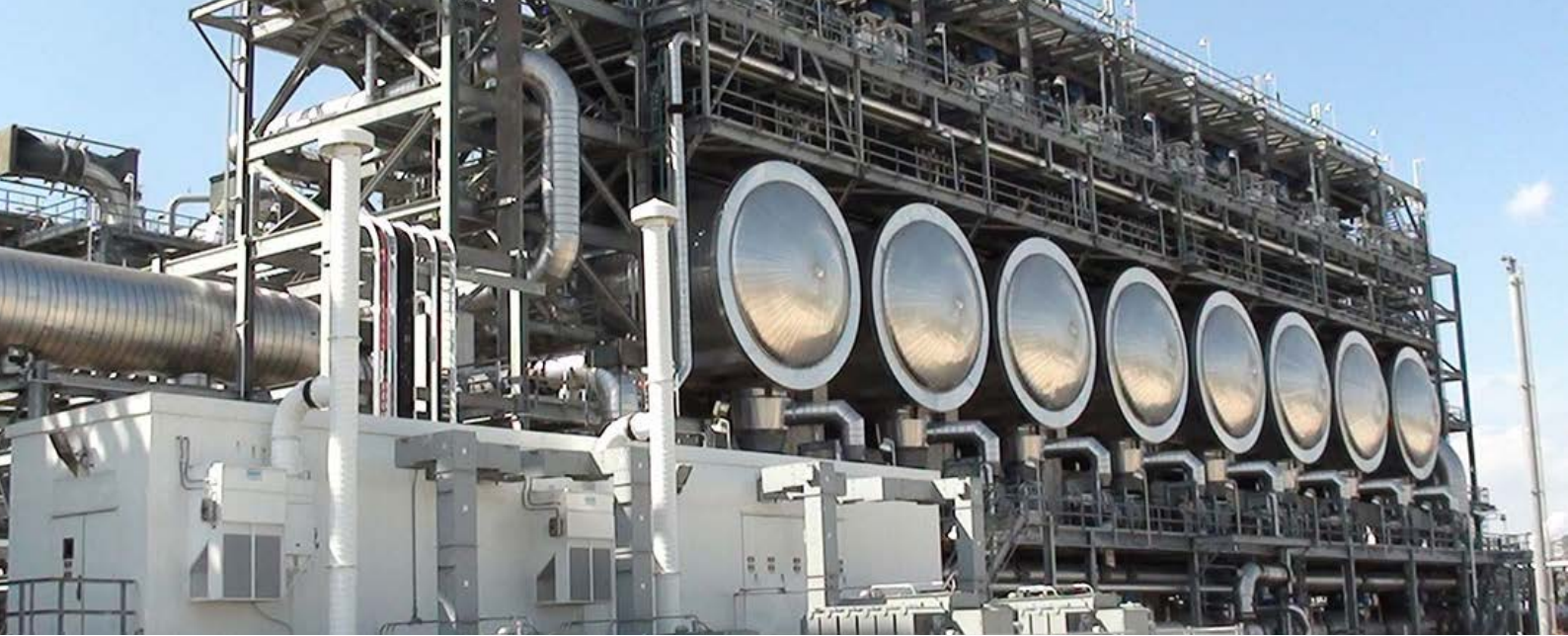
▲ Propane De-Hydrogenation(PDH) Plant View
